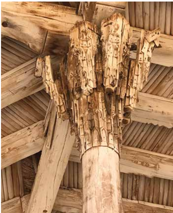
Figure 12. Beamed ceiling of the Langar Ota mosque. Although the structural wood is stable, decorative elements such as the original fifteenth-century multicomponent carved wood capital in the exterior portico of the mosque are at risk of collapse due to water damage from rain and winter snows at the shrine in its isolated location in the mountain village of Langar Ota.
