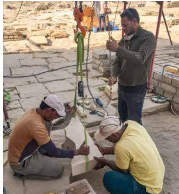
Figure 3.54. Restoration of the ancient paving around the Great Temple, February 2018. Intricately cut pieces were inserted to preserve as much of the original stone as possible. Photo: F. Helmholz.
