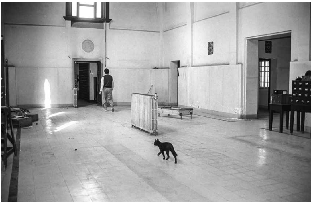
Figure 12.39. The library emptied of contents in preparation for construction, 1992. Photo: D. Darnell.
