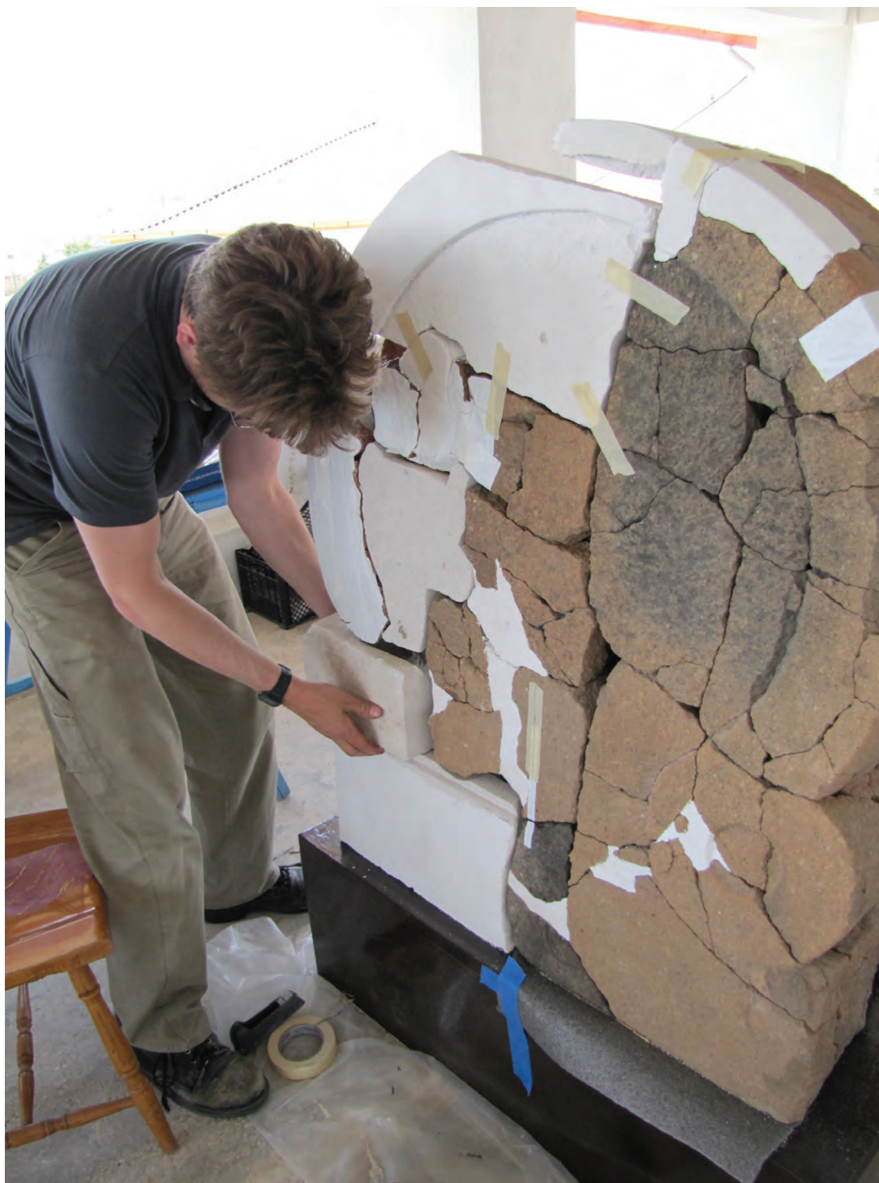
Erik Lindahl restoring Idol Block 2, KO5.232, on balcony of Kerkenes Stone Workshop in 2010. AKG gazbeton (autoclaved aerated concrete blocks) were cut to shape, as seen at top and bottom left, before Polyfilla patching plaster was employed for gapfills.
