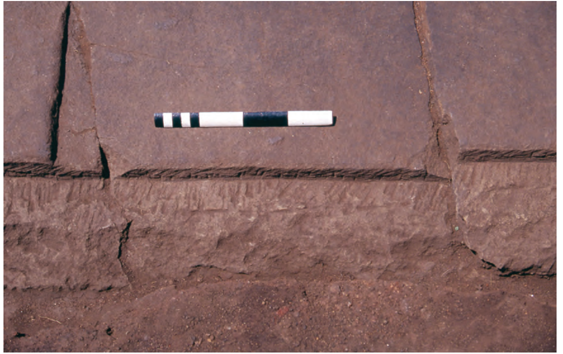
(a) Flange on the sandstone paver in front of the threshold in the central wall, with the step indicating the position of the door |
