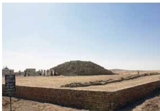
Figure 20. Backfilling operation in progress to protect the chapel remains, with the new protective wall in the foreground; view to the southwest
