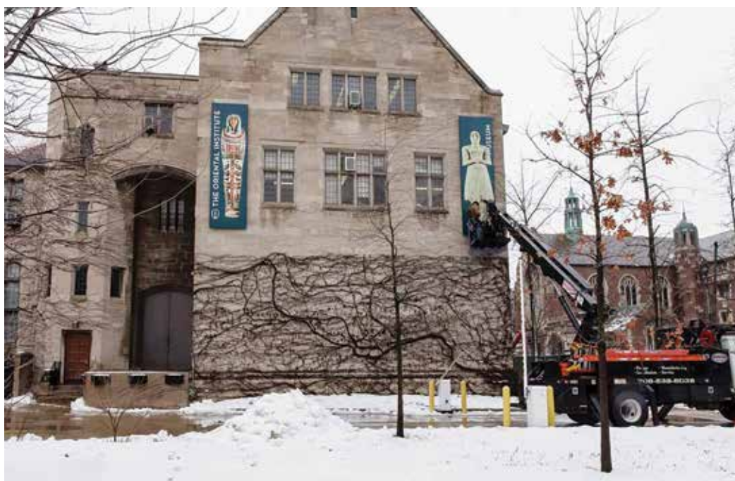
Figure 1. Installation of the new Oriental Institute banners on the east side of the building (facing Woodlawn Avenue) in February. Photo by Anna Ressman
