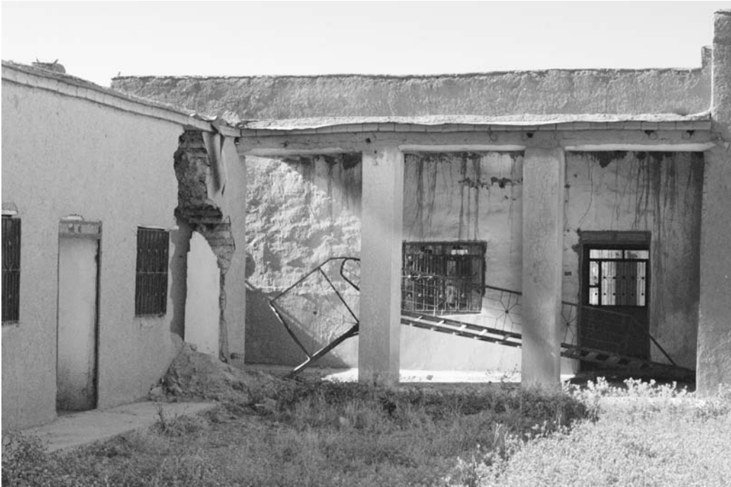
Figure 3. Living quarters and main work room of the Hamoukar dig house, built in 2000 and 2001 by MacGuire Gibson. Photo shows damage to a doorway and the roof
