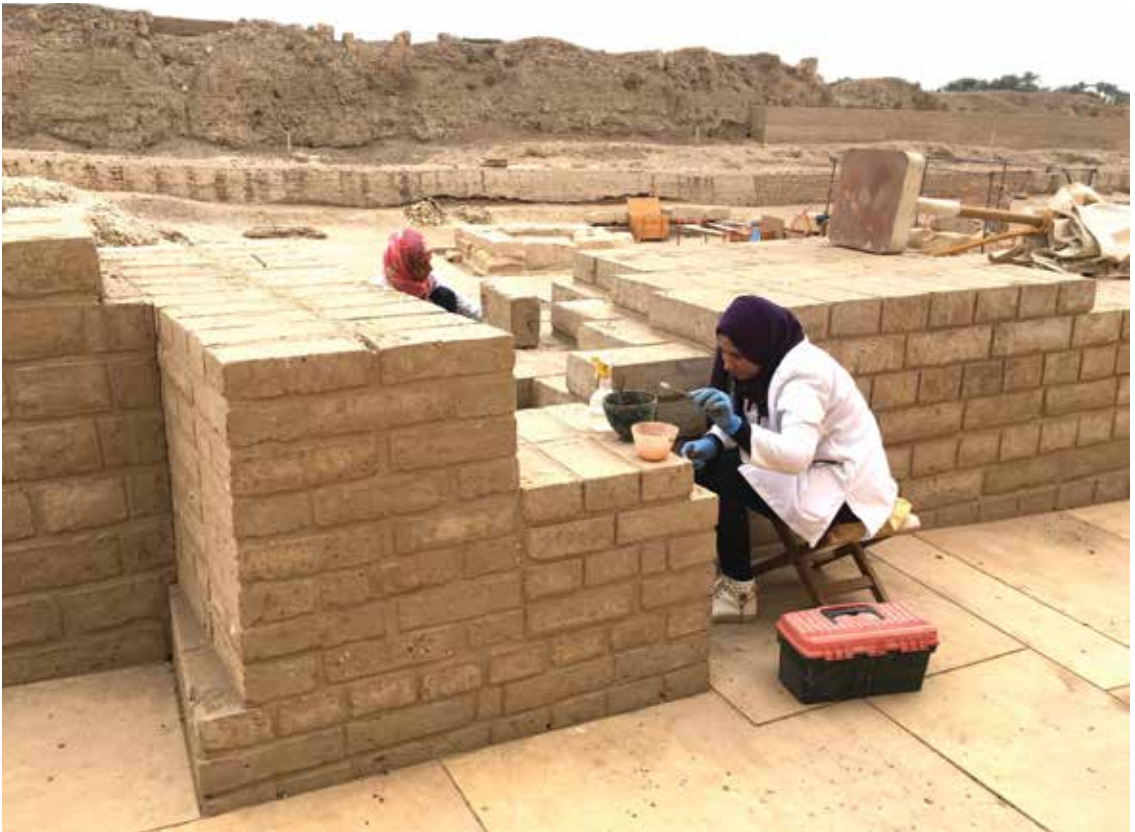
Figure 13. Finishing the restored mudbrick wall of Ramesses III. Photo by Ray Johnson.
