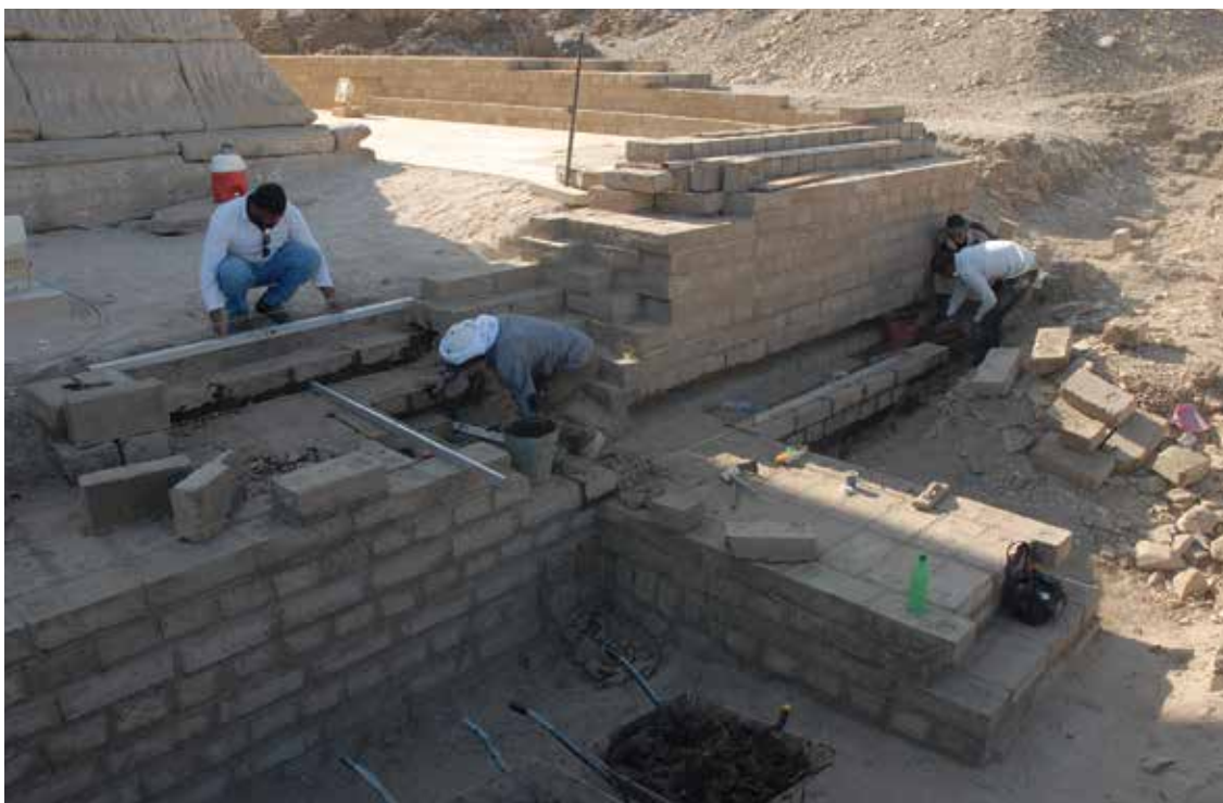
Figure 7. Conservation team restoring mudbrick walls at the northwest corner of the Ramesses III mortuary temple. Photo by Mohamed Abo el-Makarem.
