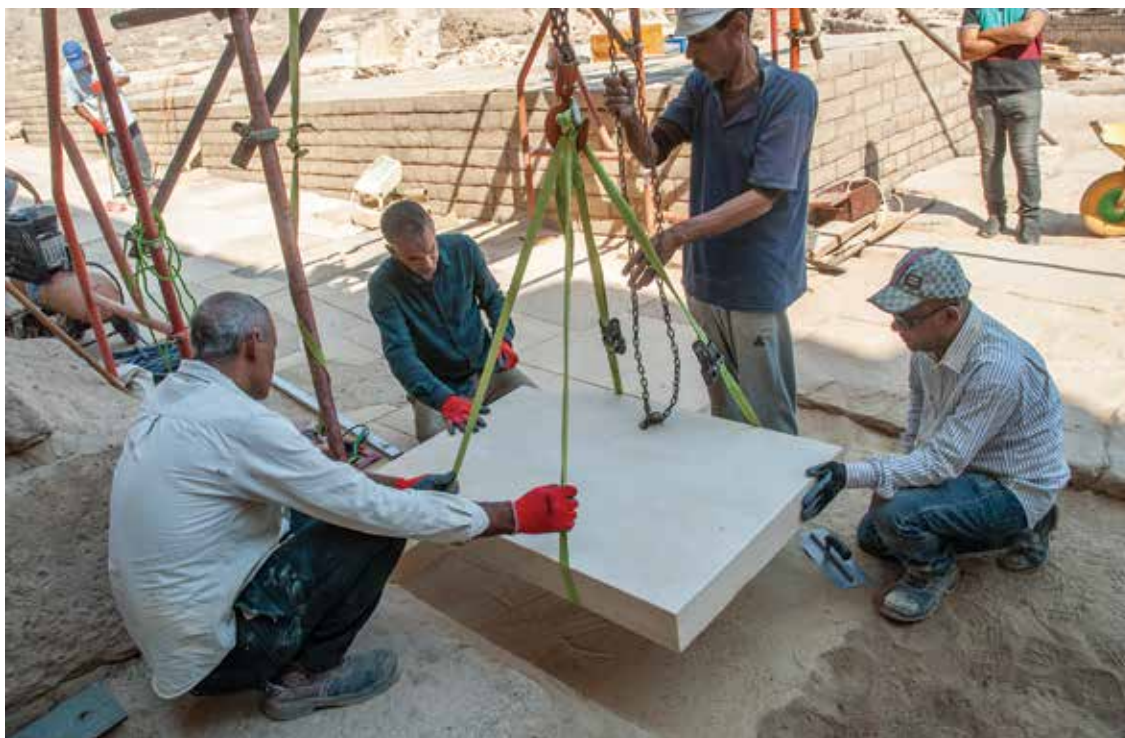
Figure 6. Stonemasonry team installing new sandstone paving block in the north sector of the Ramesses III mortuary temple. Photo by Frank Helmholz.
