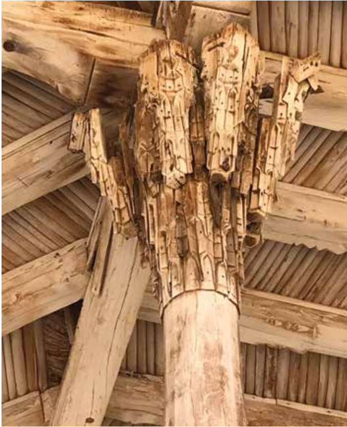
Figure 12. Beamed ceiling of the Langar Ota mosque. Although the structural wood is stable, decorative elements such as the original fifteenth-century multicomponent carved wood capital in the exterior portico of the mosque are at risk of collapse due to water damage from rain and winter snows at the shrine in its isolated location in the mountain village of Langar Ota.
