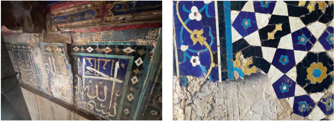
Figure 5. Panels and pieces of tile detaching from the walls, and in some cases partially collapsing, due to water damage to the calligraphic and geometric registers.
