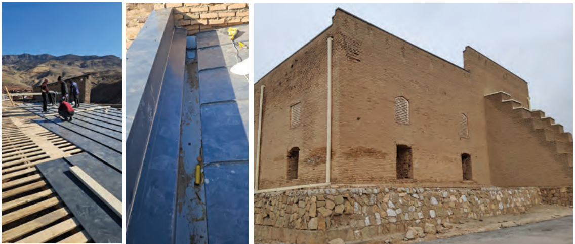
Figure 6. Installation of the new steel roof, steel-sheathed gutters, and drainpipes with extenders to carry water away from the mosque's stone foundations.
