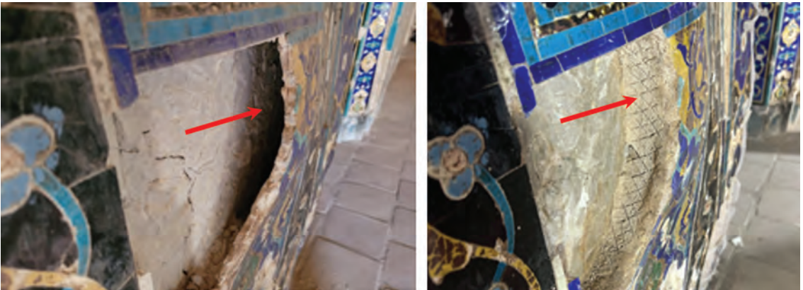
Figure 9. Stabilization of sections of loosened tilework by infilling the voids behind them with sponges soaked in consolidants, then sealing them with mortar made from traditional building materials.
