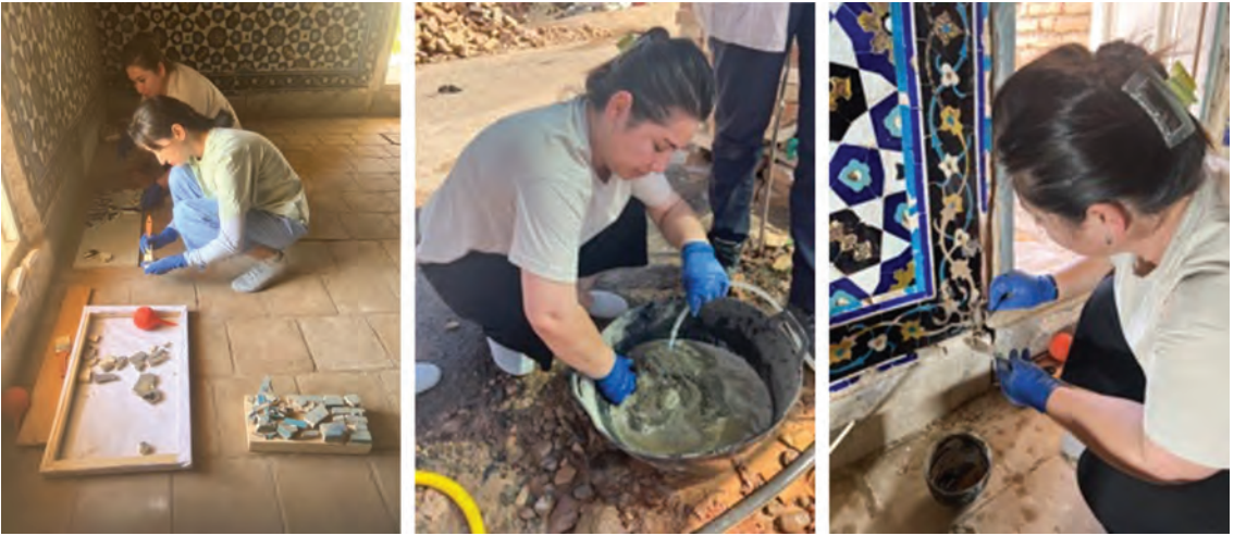
Figure 8. Uzbek conservators Malika Beknazarova cleaning individual cut-tile pieces (left) and Nargiza Kalandarova mixing mortar from traditional building materials and inserting it to repair the geometric tile register (center and right).
