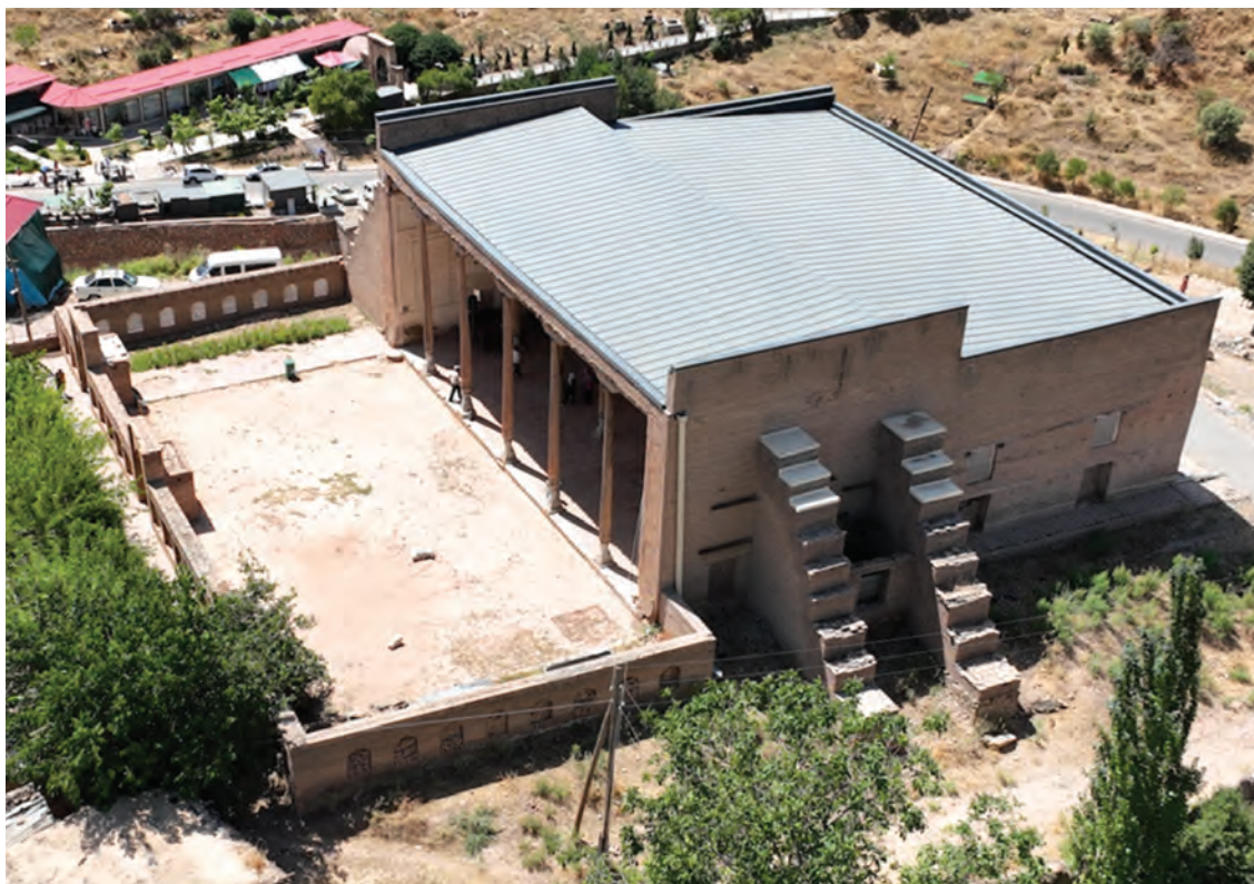
Figure 7. The Langar Ota mosque with its new steel roof, drains, and metal rain caps on the buttresses.
