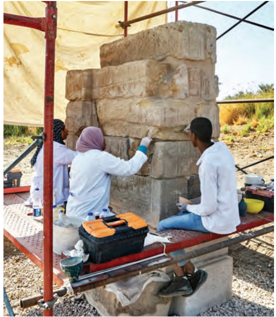
Figure 6. Conservation team finalizing restoration of the Claudius Gate. Photo by Yarko Kobylecky.
