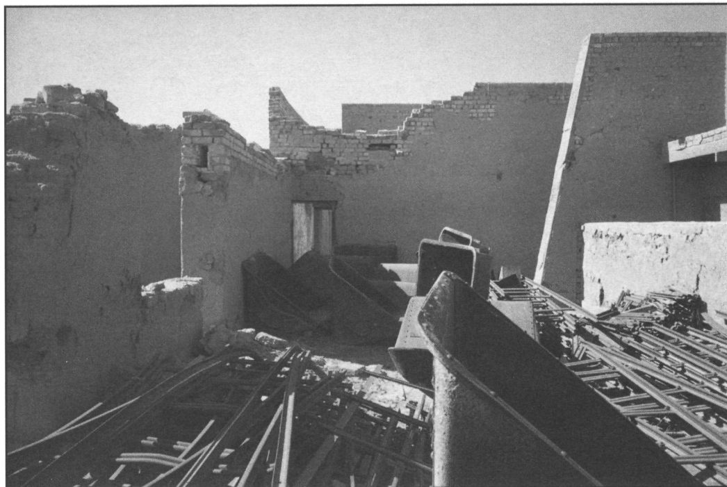
Expedition house at Nippur, damaged portion
