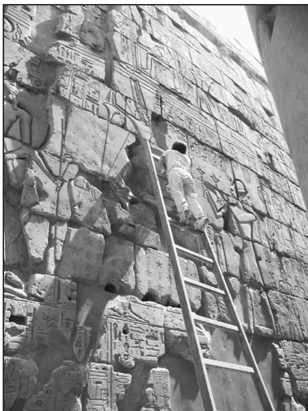
Figure 12. Hiroko installing a plumb bob monitor halfway up the south face of the east pylon, Luxor Temple. Luxor, Egypt. Photograph by Ray Johnson
