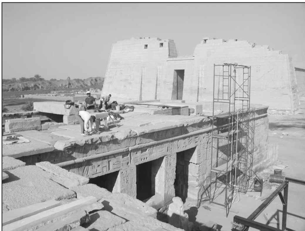
Figure 6. Dany Roy and Chicago House workmen doing restoration work on the roof of the small Amun temple, Medinet Habu. Digital photograph by Ray Johnson
