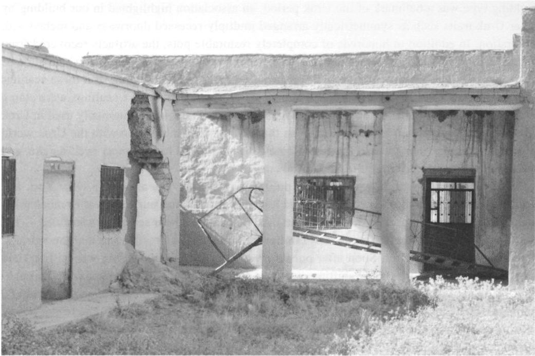
Figure 3. Living quarters and main work room of the Hamoukar dig house, built in 2000 and 2001 by MacGuire Gibson. Photo shows damage to a doorway and the roof
