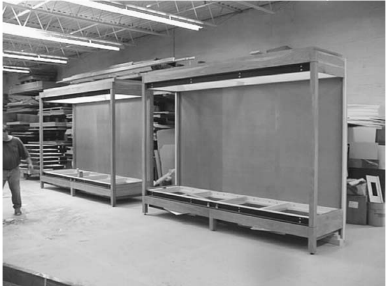
Figure 1. Display case for the East Gallery being constructed at Helmut Guenschel Company in Baltimore
