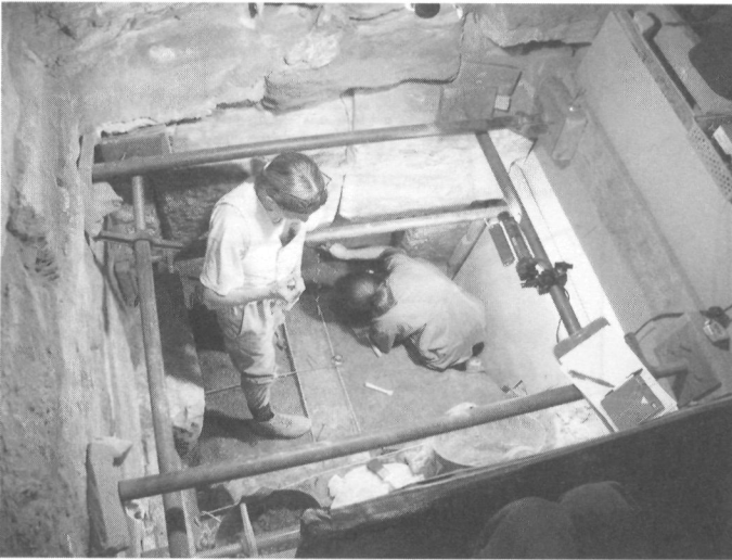
Figure 7. Recording of excavated footing of the naos in the Naos Room, small Amun temple, Medinet Habu by Lisa Giddy and Tina Di Cerbo. Photo by Ray Johnson
