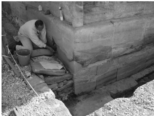
Consolidation and infilling the outer southwestern wall of the small Amun temple sanctuary. Photo by Ray Johnson
