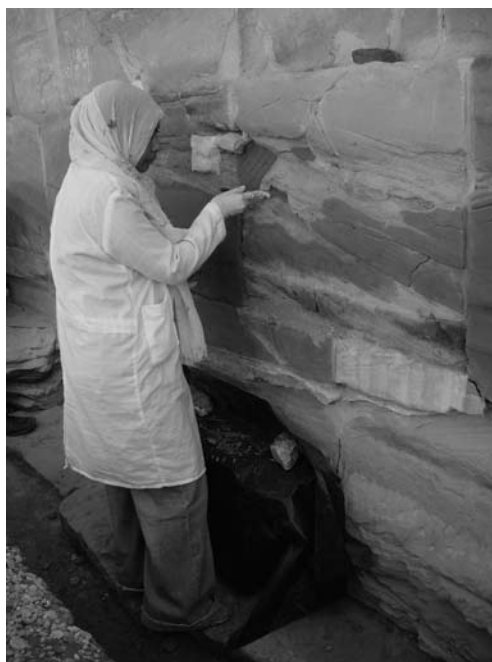
Figure 5. Conservator Hala consolidating back wall of the small Amun temple. Photo by Ray Johnson
