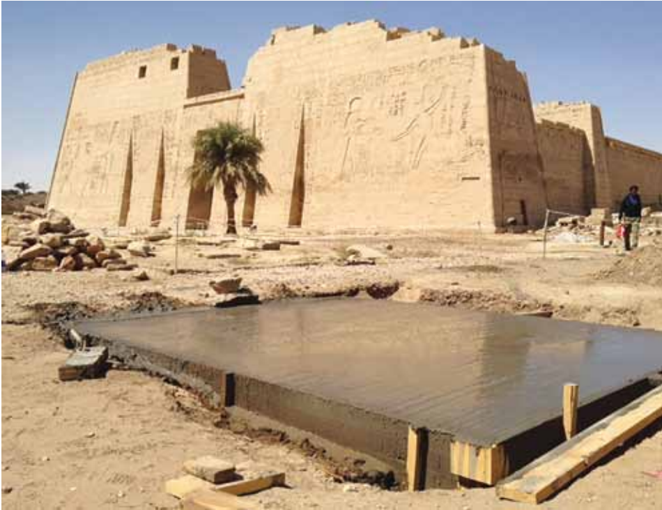
Figure 5. Poured, reinforced-concrete foundation for the Domitian gate. Medinet Habu. Photo by Frank Helmholz
