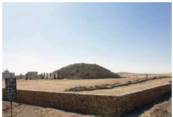
Figure 20. Backfilling operation in progress to protect the chapel remains, with the new protective wall in the foreground; view to the southwest
