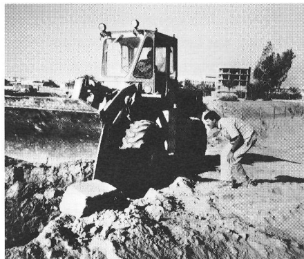
John Meloy "chasing" a bulldozer looking for archaeological layers beneath the sand; in the foreground lies debris from demolished barracks.
