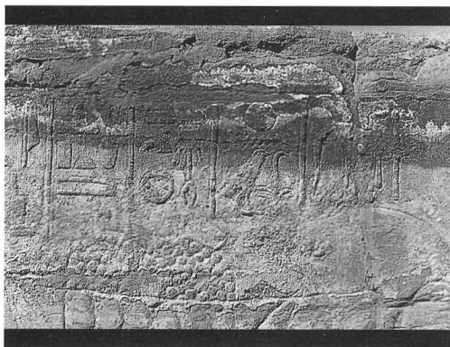
Two days after the torrential rains of New Year's Eve, salts begin to crystalize along the tops of walls at Luxor temple.
