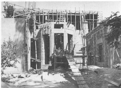
Figure 2. The expansion of the library hall, seen here during construction in August 1993, entailed the reconstruction of the art-deco alcove in roughly its original position
