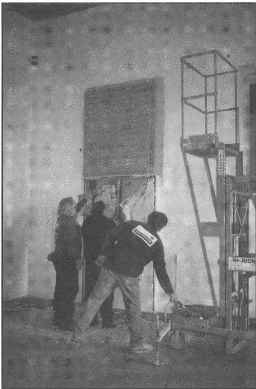
Figure 1. Doug Mertes, Milt Samuelson, and Bill Allison, Sr., from Belding/Walbridge preparing to remove an inscribed glazed brick panel from wall in order to relocate it as part of the Persian Gallery reinstatement. Photograph by Laura D'Alessandro
