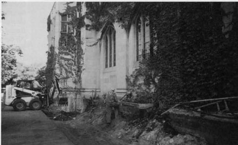
A SIGN OF THINGS TO COME—The University of Chicago has graciously provided funding for a wheelchair-accessible ramp entrance to the Oriental Institute. Construction is already well underway, with completion expected in January. Photograph by Jean Grant
