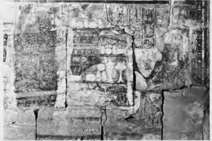
Reliefs at Medinet Habu after cleaning; compare the "before" photo of the same wall elsewhere on this page. Photo L. Bell.
