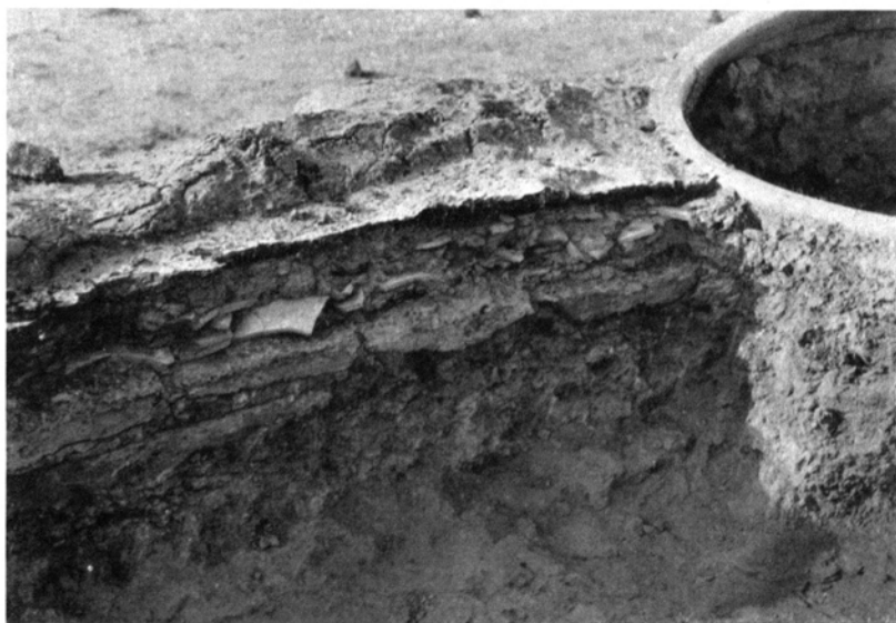
FIG. 69.—DETAILS OF THE CONSTRUCTION OF THE SHALLOW DRAIN LEADING INTO BASIN L 45:1, SHOWING SUCCESSIVE LAYERS OF BAKED BRICKS, POTSHERDS, AND, ON TOP, BITUMEN
