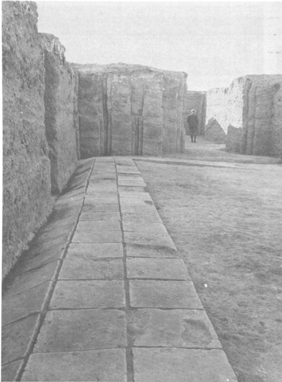
(a) Ishchali—Court 1-R.29 from the East Court of the West Unit of the North Wing Showing the Tilt in the Pavement Caused by the Wall Settling
