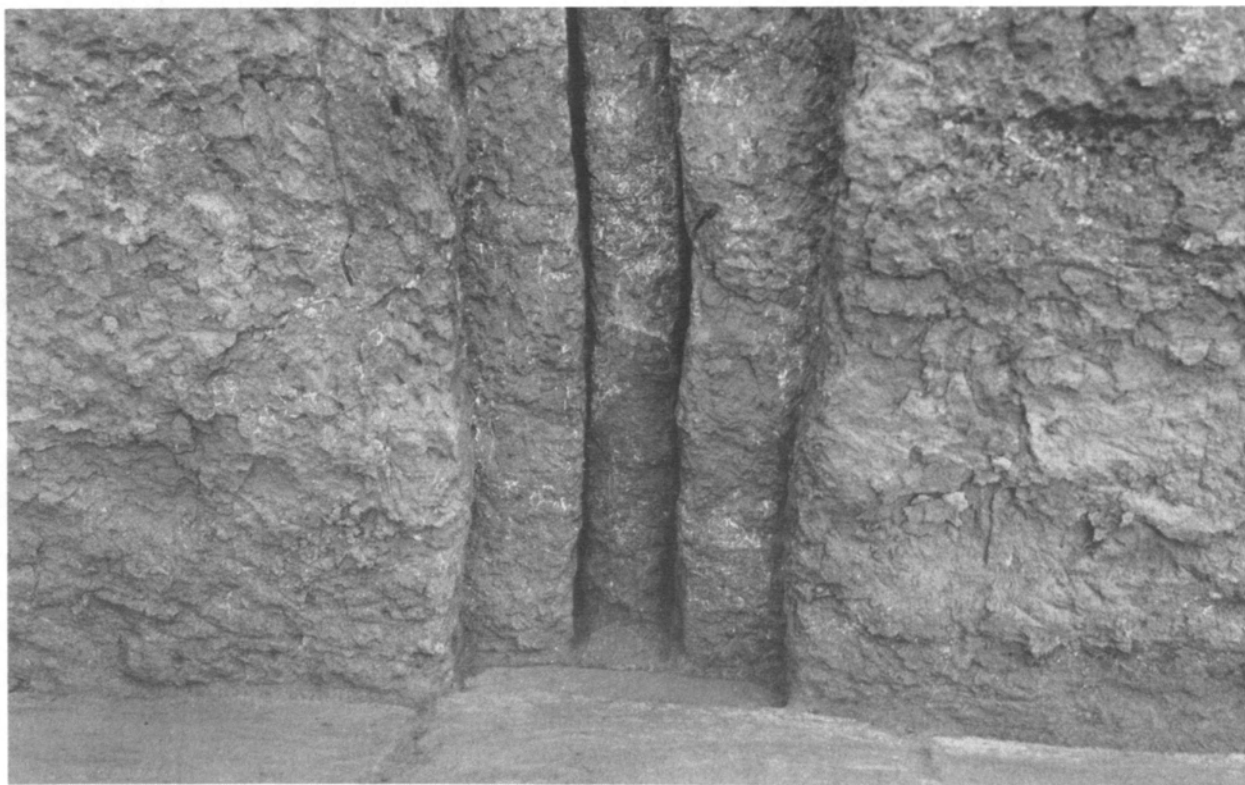
(b) Ishchali—Detail of the Recessed Wall Decoration (“Slotted Simulated Towers”) in Court 2-T.29 of Period I-A, Seen from the East
